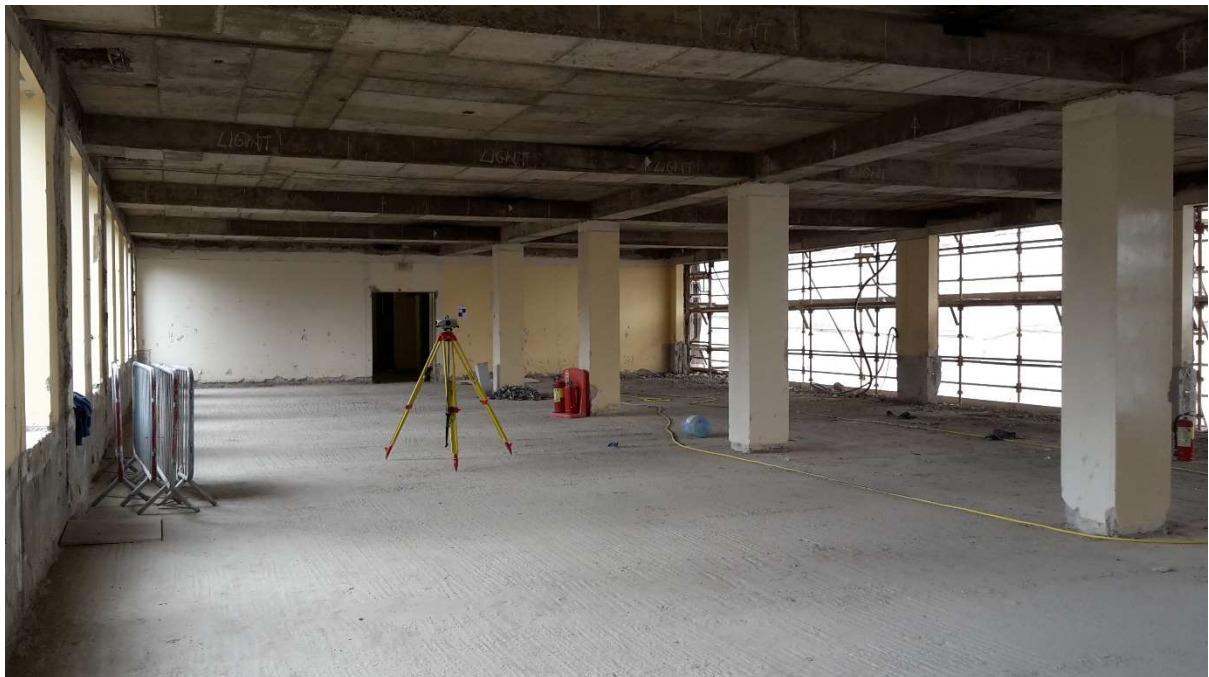
Digital levelling through a building under construction to complete a scanning project
