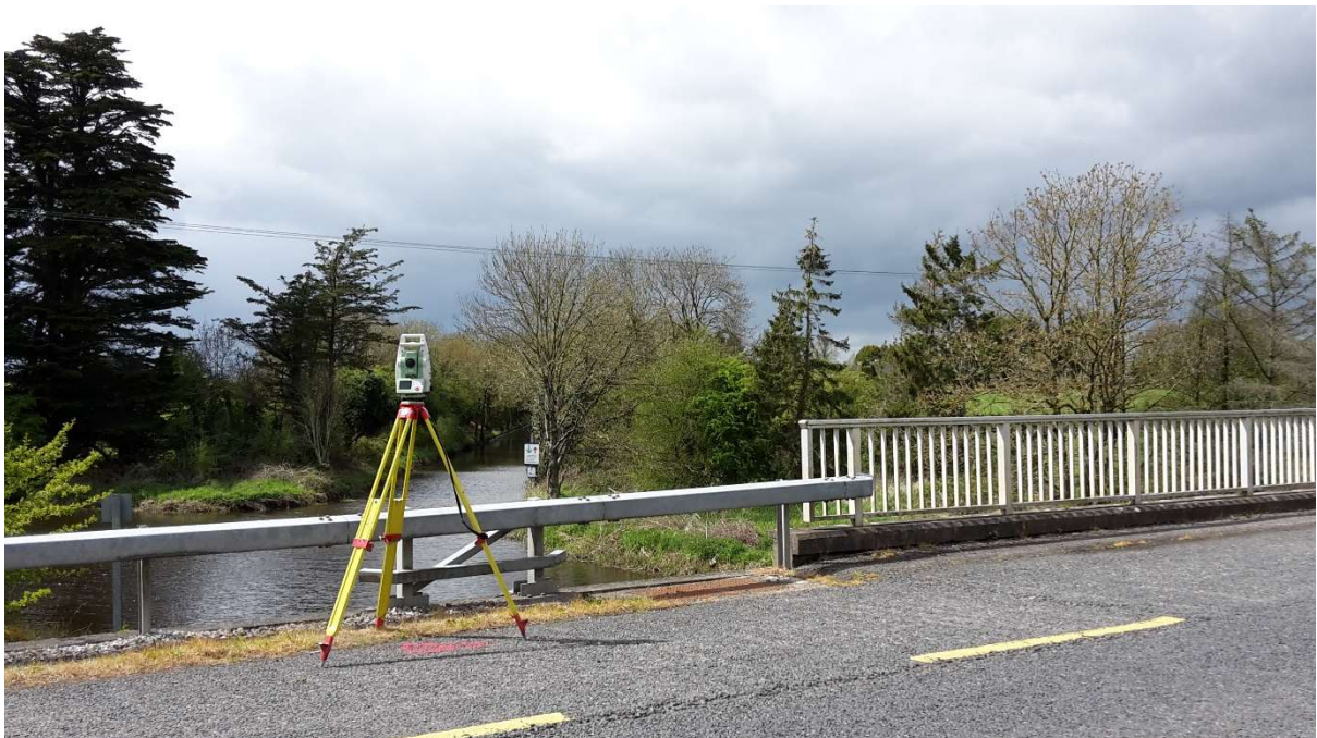
Topographic survey of a bridge and its surroundings in Cloondara, Co. Longford
